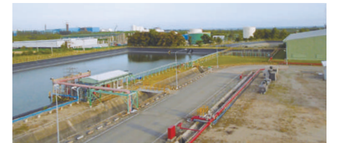
Rainwater is collected and used to provide industrial water to neighboring partner companies (Asia Silicones Monomer Limited)
